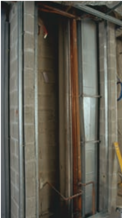
SERVICE SHAFT WITH PERIMETER ANGLE FRAME FIXED
