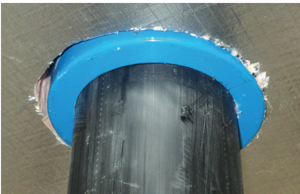
Figure 7 Penetration example - Kingspan Kooltherm® K10 PLUS Soffit Board installed tight around the fire collar and HDPE service pipe.
