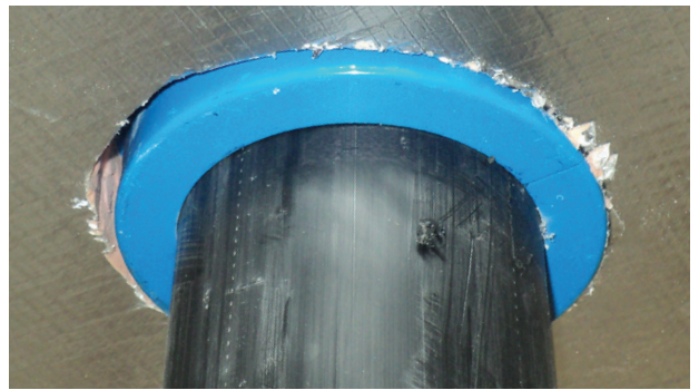
Figure 7 Penetration example - Kingspan Kooltherm ® K10 G2W White Soffit Board installed tight around the fire collar and HDPE service pipe.
