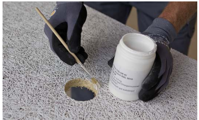
Edge touch-up – Cover cut edges with paint if these are not concealed by a cover.
